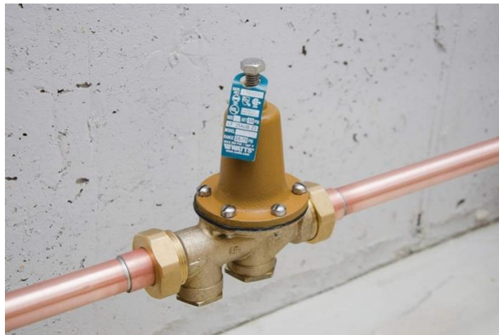
Figure 1 - Watts LF25AUB-Z3 water pressure regulator installed in residential water pipe (water flows from left to right)
